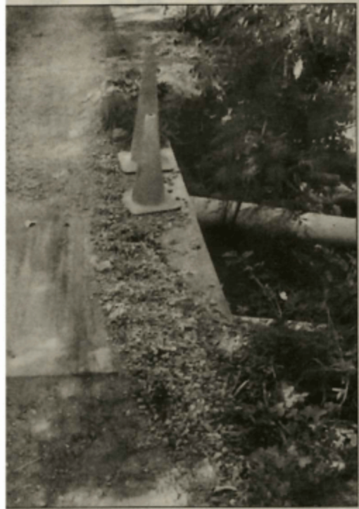
John is currently mitigated with a steel plate. The asking to rehabilitate sections of the road.
