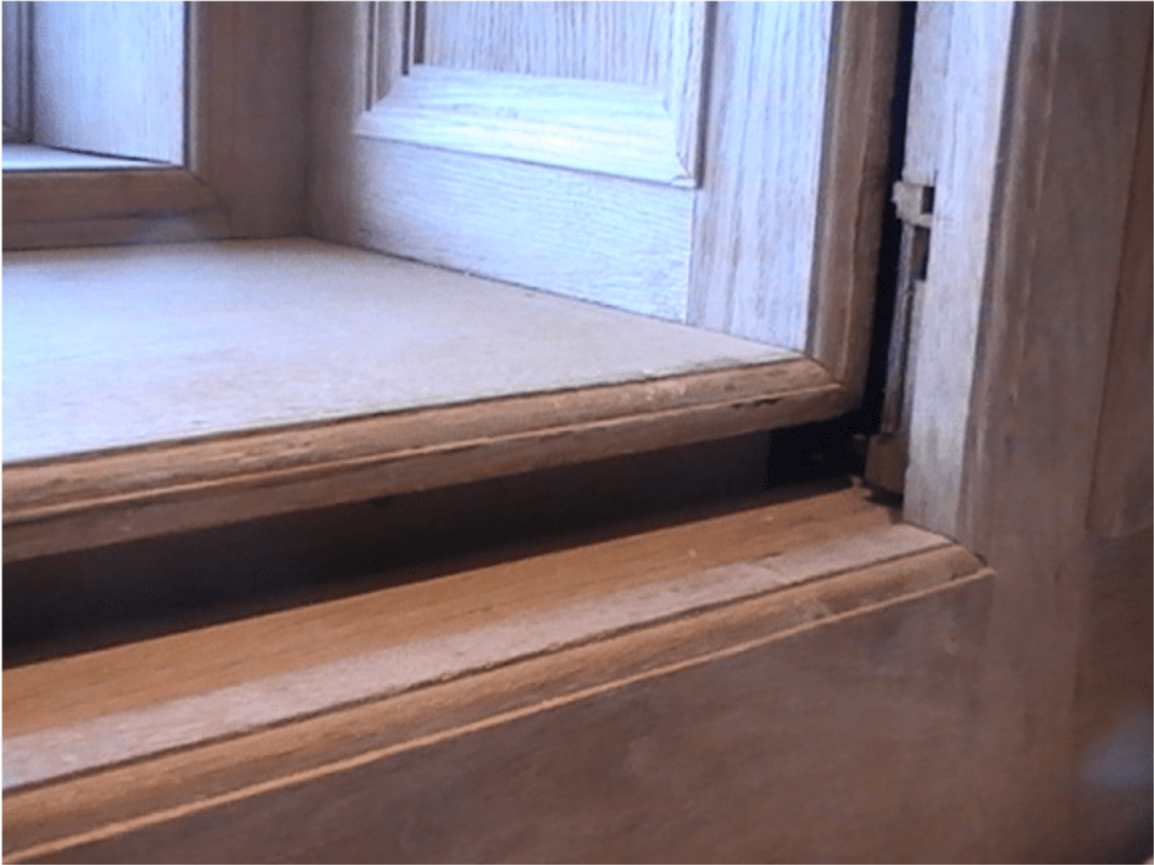
Edges of wood discolored, chipped. Enormous gap between window frame and outside frame. Unfinished appearance.
