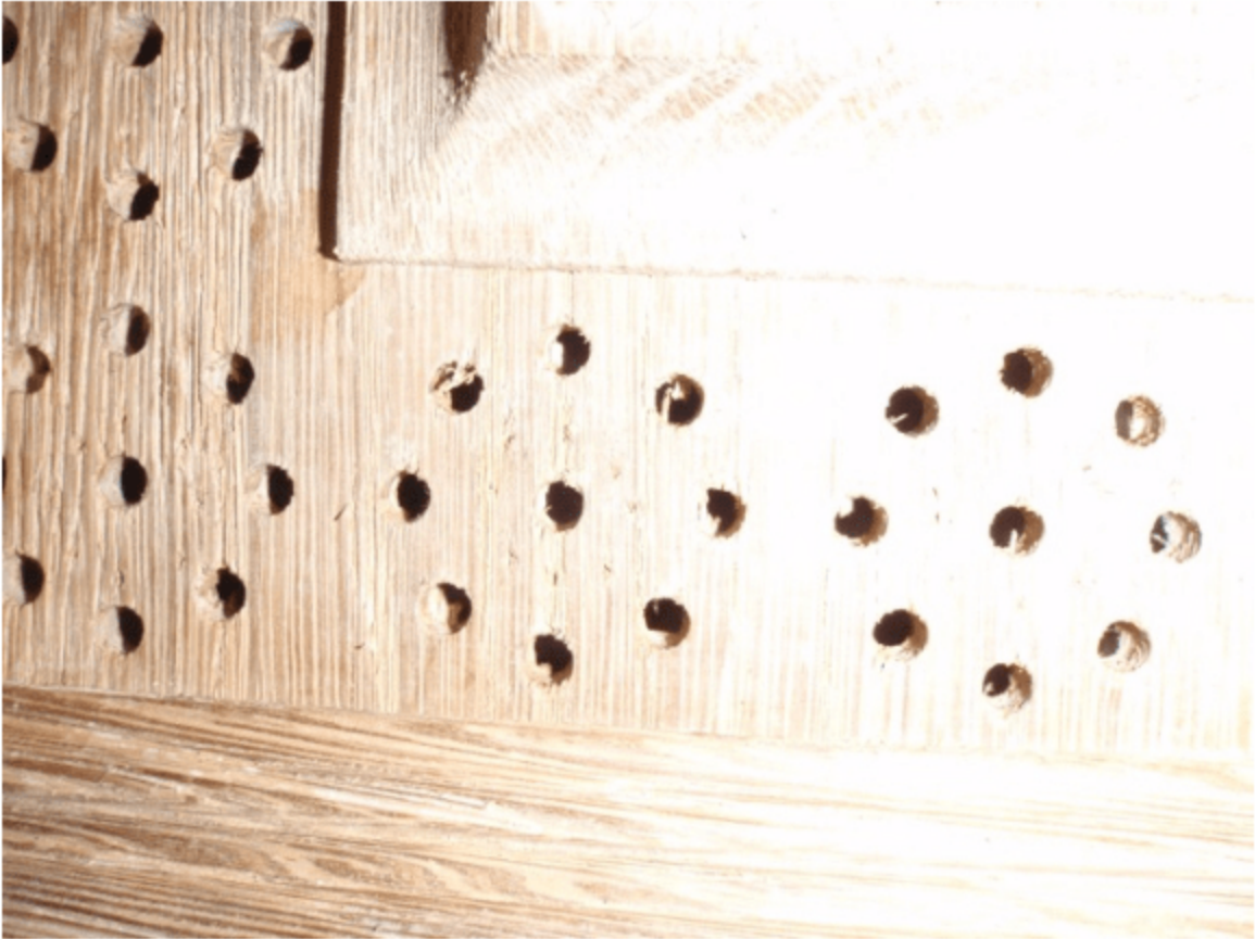
Unsanded holes. Rough unfinished appearance.
