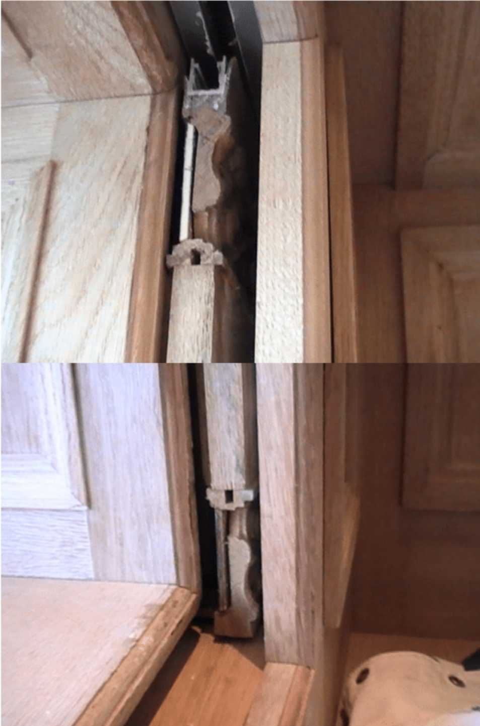
Shoddy workmanship. Edges and surface of wood rough and uneven; discolored and unfinished appearance.
