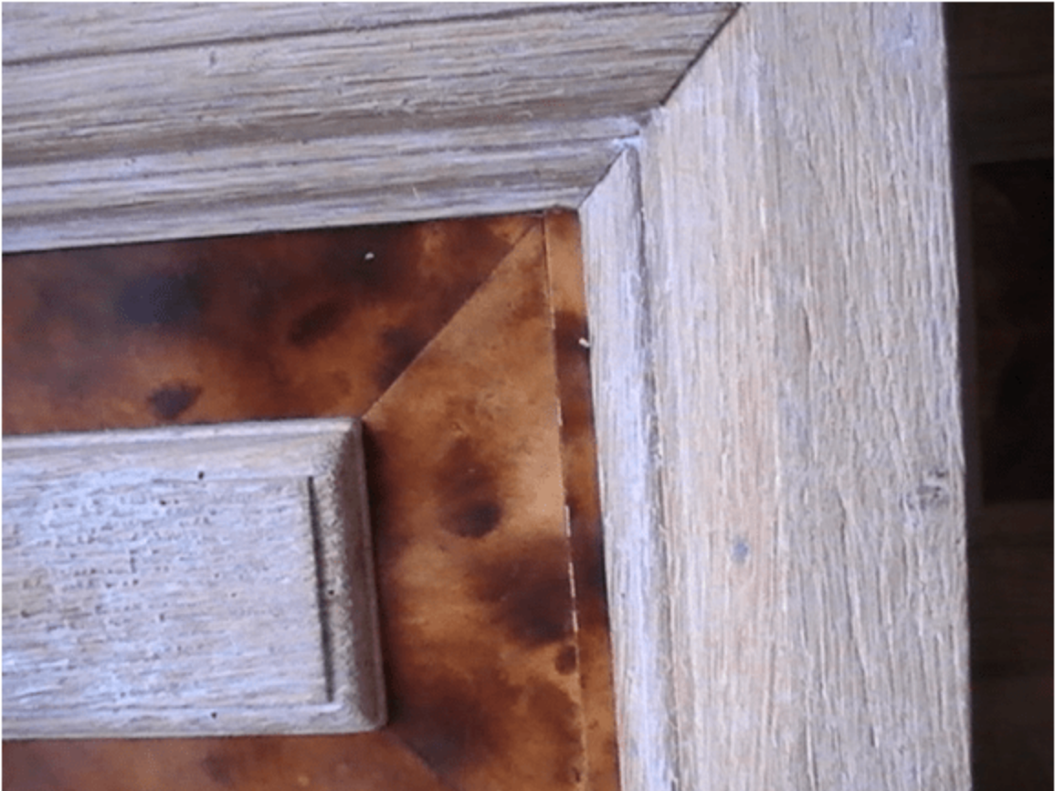
Rough, pockmarked wood with no apparent or poor finish. Tortoise Shell application patched and chipped.
