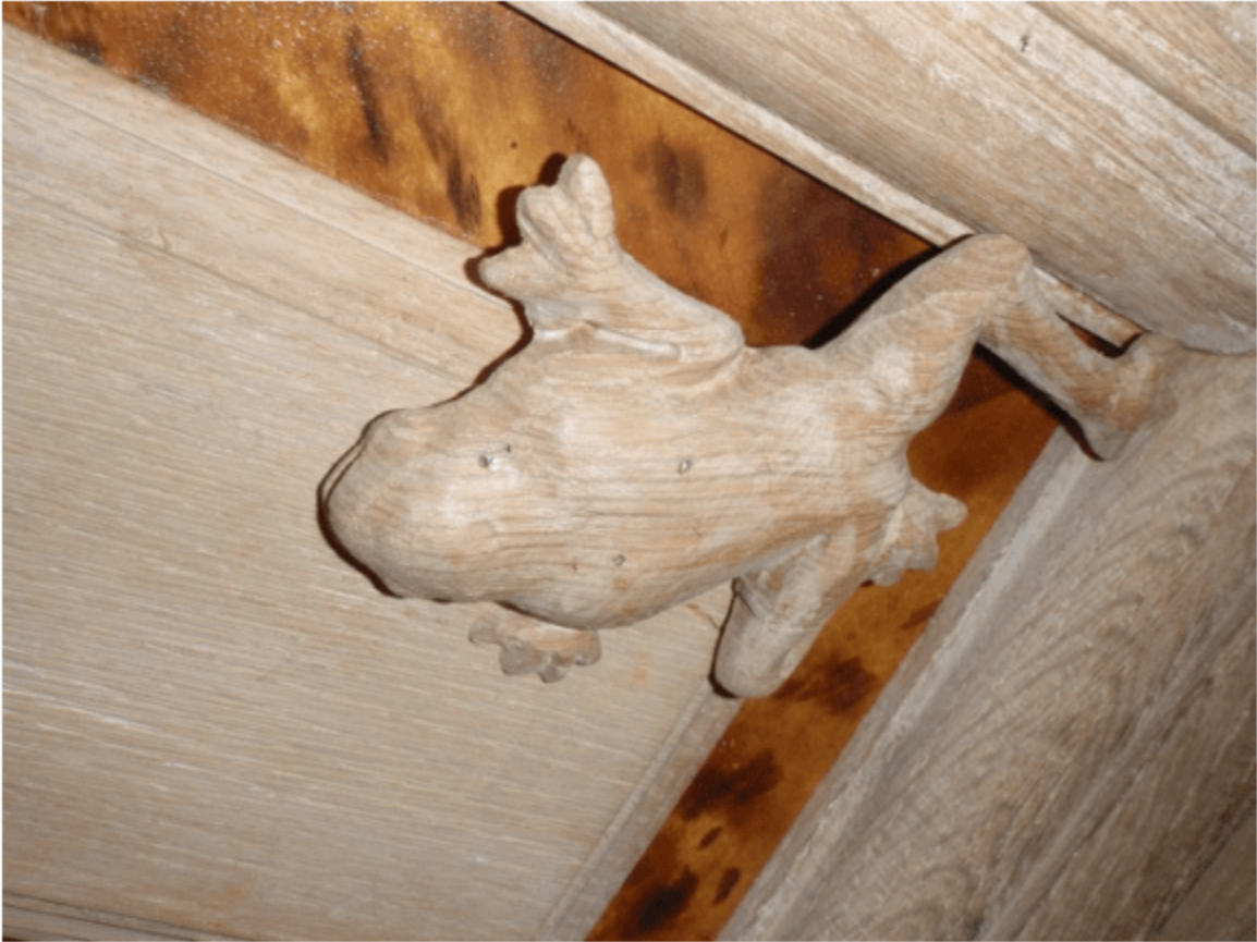
Nail holes in frog carving. Uneven application of color to frog and wood work.
