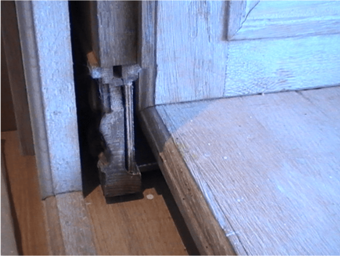
Shoddy workmanship. Edges and surfaces of wood rough, uneven, chipped and cracked. Discoloration and unfinished appearance.
