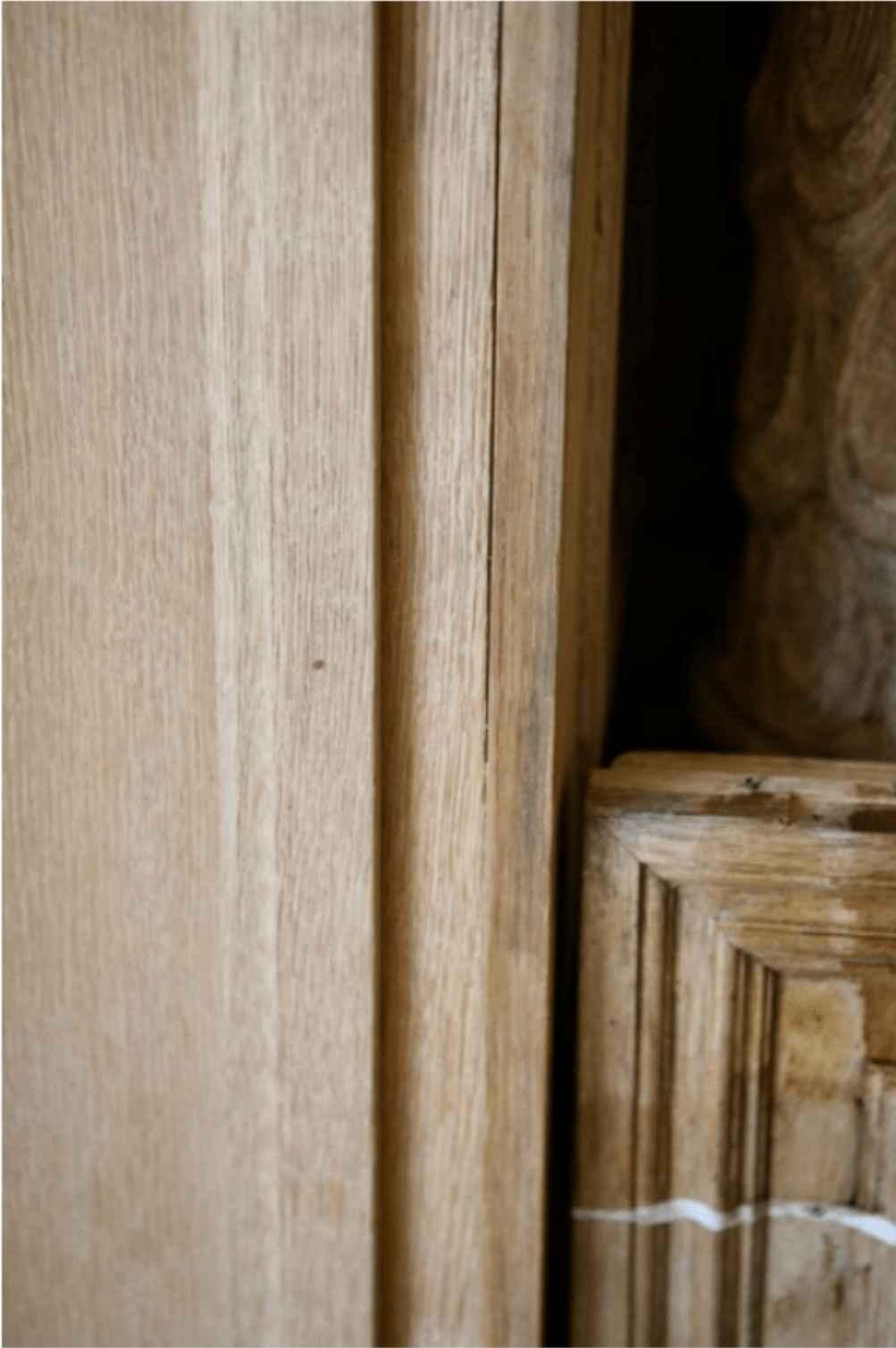
Discoloration, white stripe of foreign material evident, uneven application of stain.
