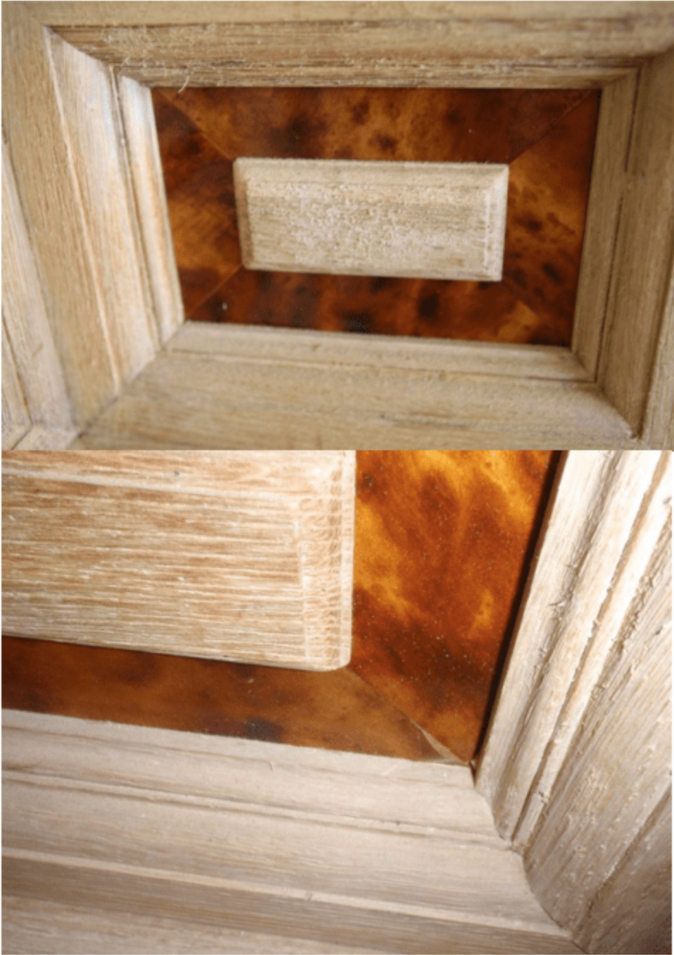
Splintery, rough and pocked wood, uneven application of stain, and apparently no finish in many places. Tortoise shell application marred at bottom right hand corner of bottom photo.
