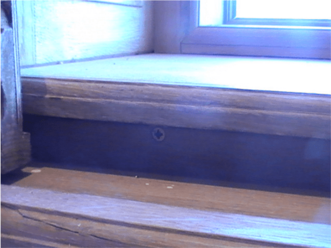
Cracked wood. Rough unfinished edges and surfaces. Screw apparent. Gap between Window frame and outside frame. Discoloration.
