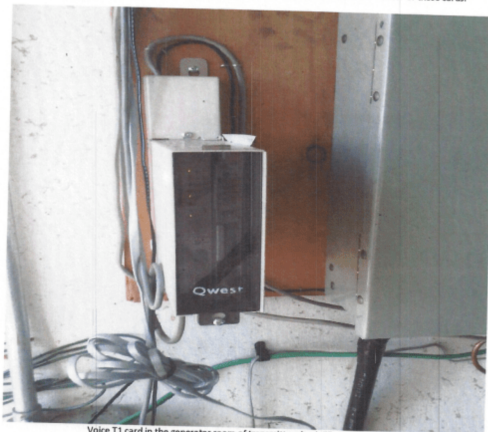
Voice T1 card in the generator room of transmitter shack 75 at Sandia Crest.
