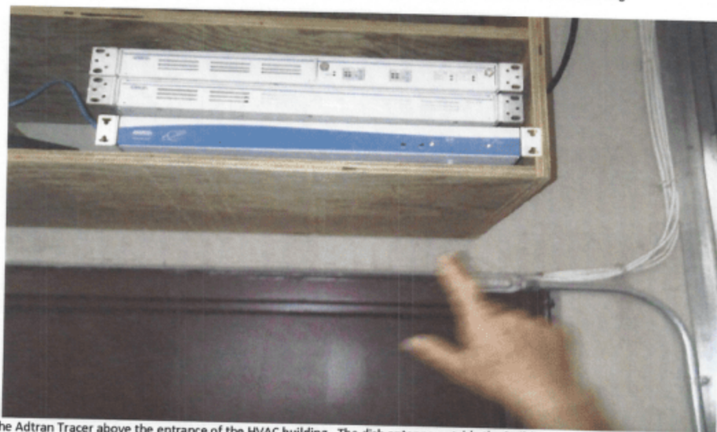
Wireless signal from Sandia Crest is received at this dish antenna outside the HVAC room at Zorro Ranch. The black coax cable running down the pole connects to the companion Adtran Tracer above the entrance of the HVAC building.
