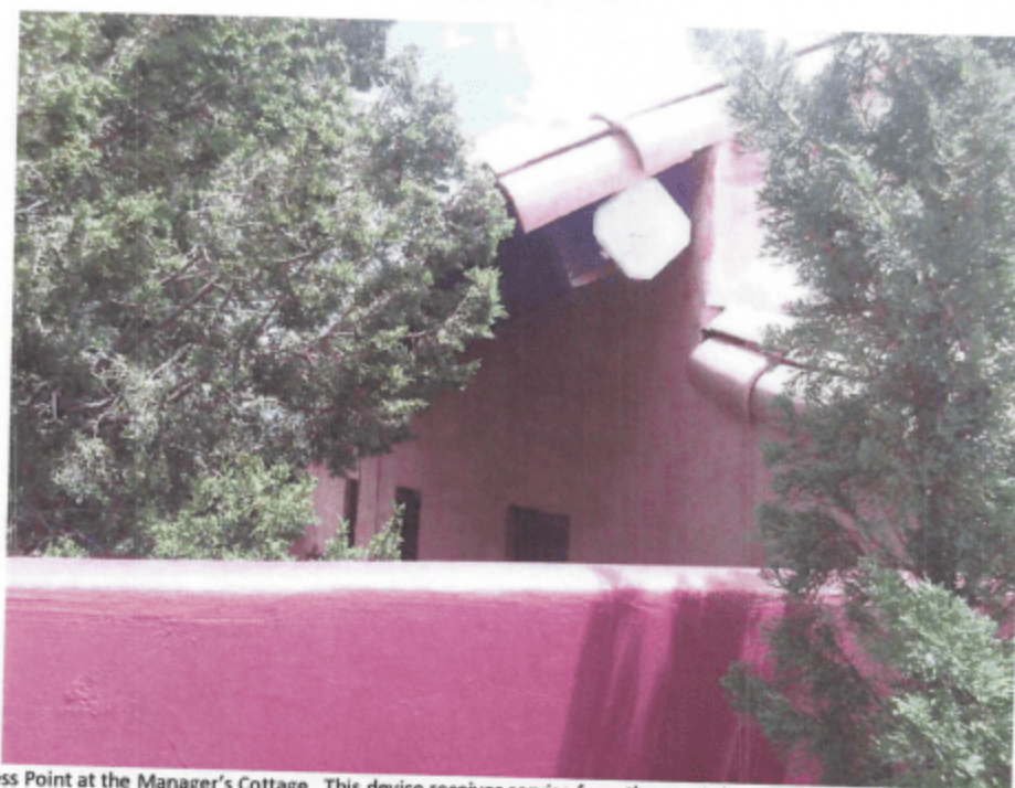
Lodge Wireless Access Point located at the apex of the roof. This device receives service from the omni-directional antenna above the entrance of the HVAC building.
